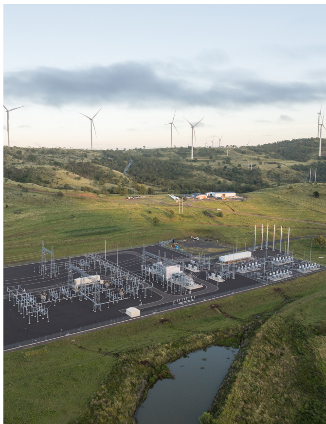
Image courtesy of Powerlink.
