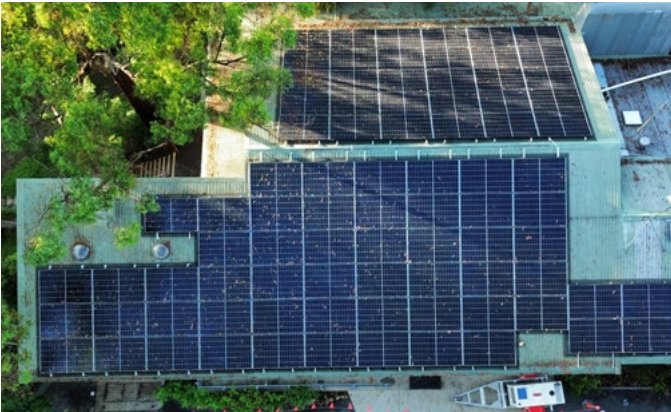
Numinbah Valley Environmental Education Centre - Solar Upgrade Installation. Image courtesy of the Queensland Government.
